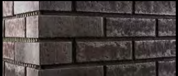
The finished joint pattern. Full masonry stretches are grouted at one go.
