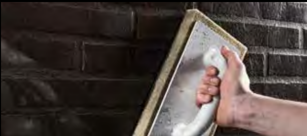
The excess grout is washed off diagonally using a plaster float with a sponge or foam pad.
