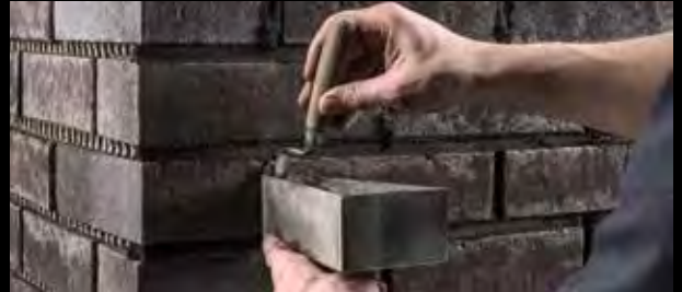
The vertical joints can be finished more easily with a smaller pointing trowel.
