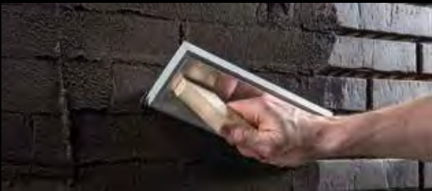
With the slurry method, the joints are filled diagonally with the grouting or plaster float. Walls should be worked from top to bottom.
