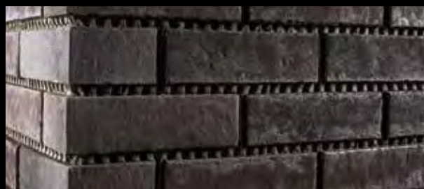
The finished surface. Grouting can be done after the appropriate drying time.
