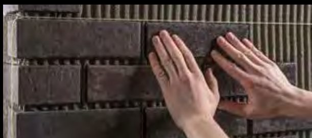
Use a string to plumb the clinker area. The clinker slips are pressed into the adhesive bed.
